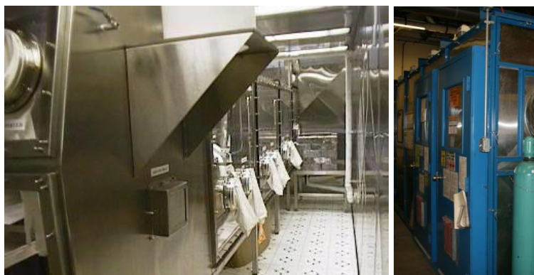
Multiport glovebox facility (left) housed in a 20'x24' Permacon Rad facility (right) with 3 stage HEPA filters.
